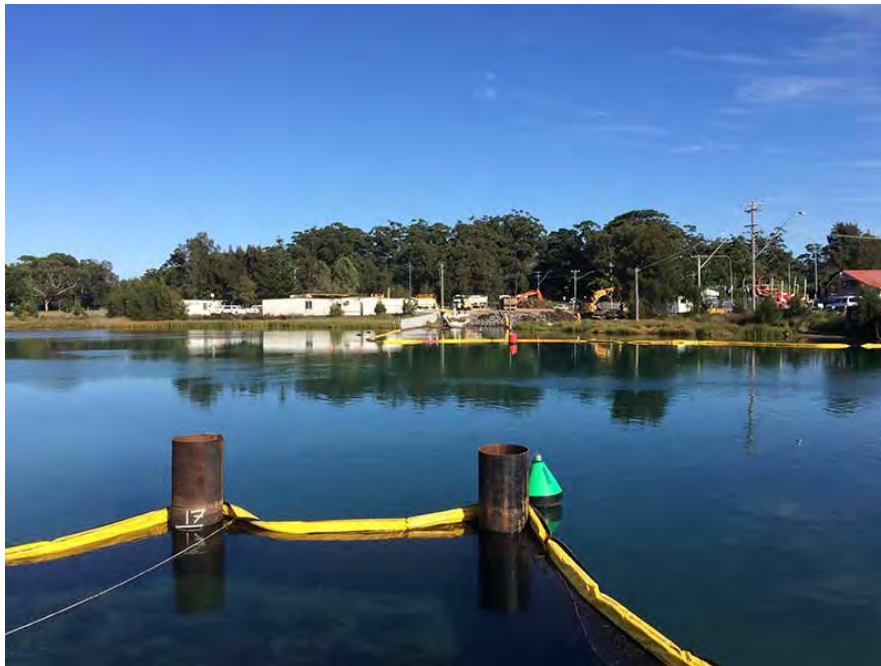
Looking south, the first pylons for the temporary bridge constructed in the channel.
